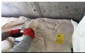
Roof Fire Blanket Joint
